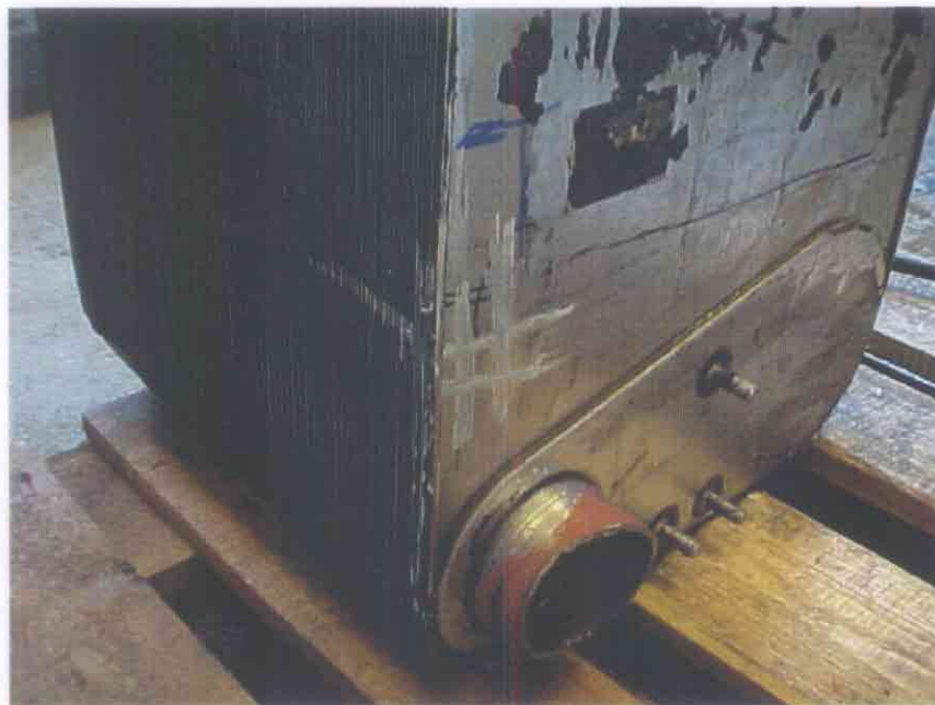
FIGURE 2 – An internal leakage in the heat exchanger was detected near porthole T4, i.e. near the pressure plate outlet of superheated vaporised refrigerant. This position corresponded to the observation of a bulge on the outside of the heat exchanger, see the white markings.
