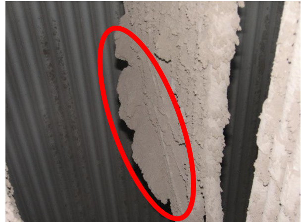
Figure 11 Picture of the ash build up on the SH3 tubes seen from the top, showing large chunks of ash deposits on the front side of the tubes facing the flow.
