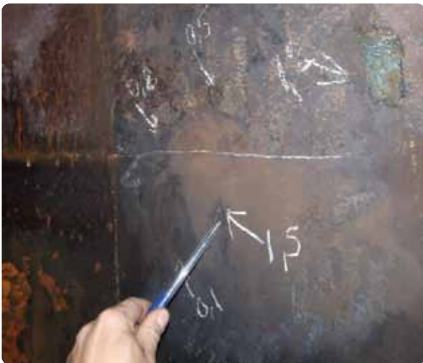
After removal of corrosion, shape and depth of the attack is assessed
