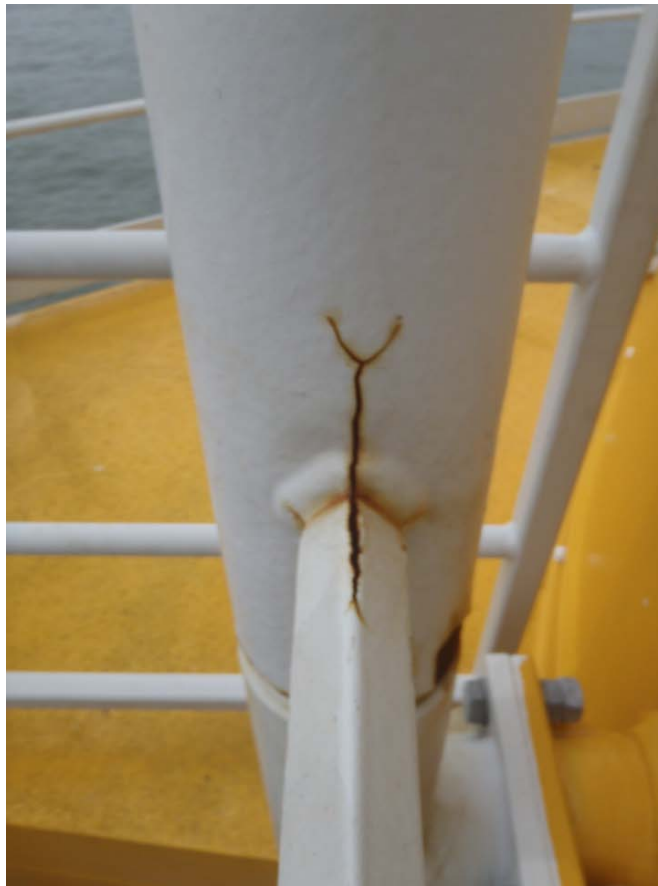
Photo 3 Cracks created by inner tension in the coating film give access to corrosion attacks.
