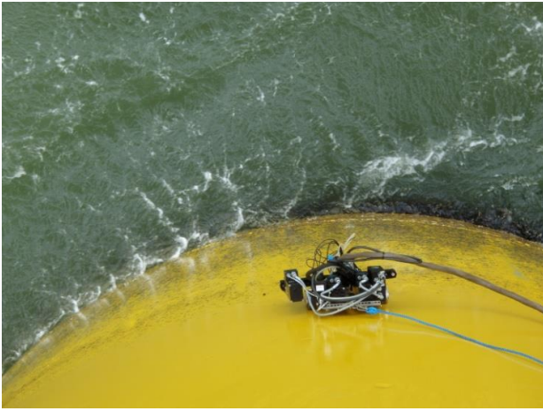
FIGURE 7: Thickness measurement by UT-crawler on the external side of transition piece by remotely controlled equipment.
