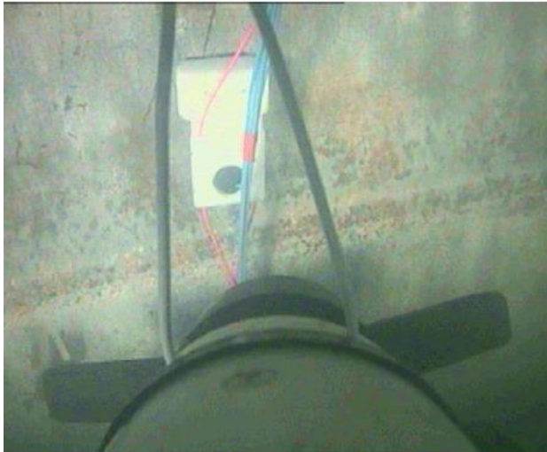
FIGURE 14: Magnet mounted zinc reference electrode seen from the actuator used for installing the probe inside the monopile.
