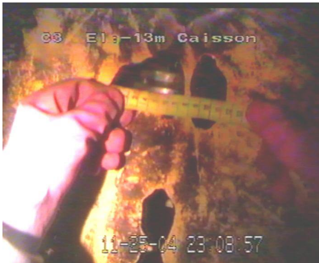
Figure 2 Measured extent of the corroded area
