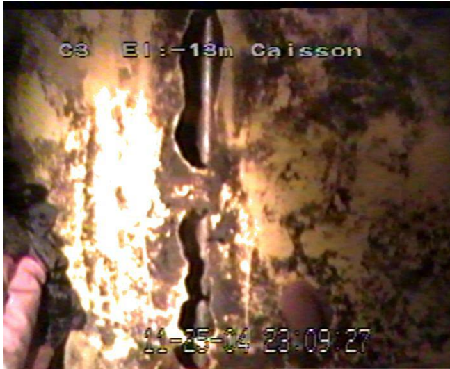
Figure 1 Corroded area after cleaning off the shells and growth
