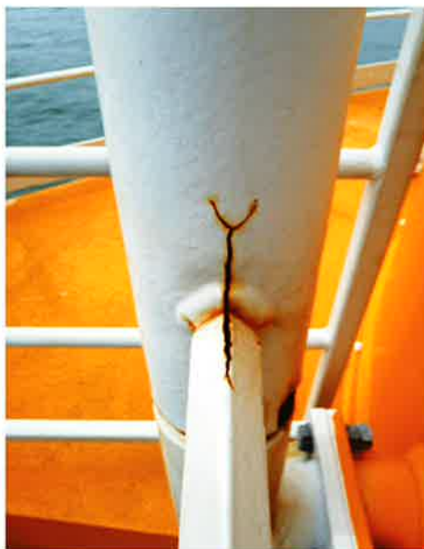
Fig. 9: The flaking of the topcoat and the penultimate intermediate coat on this boat landing was caused by aluminum dust originating from an adjacent thermal spray application during construction and from exceeding recoating intervals. Photo courtesy of FORCE Technology
