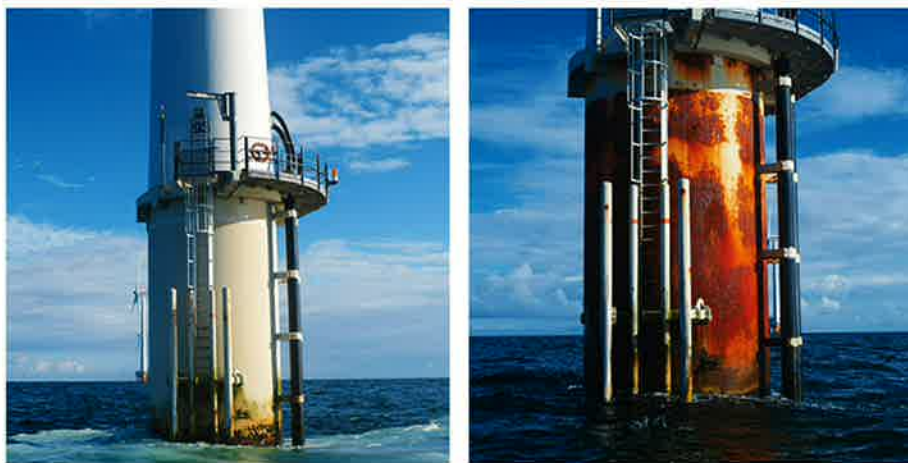
Fig. 5 (left): The two-coat epoxy system at 1,000-1,100 µm DFT on the last five of the HR1 TPs has shown good and lasting resistance, apart from damage caused by impact from supply boats, and the protection remains intact today. Fig. 6 (right): This photo shows the corrosion attacks in 2015 on TPs coated with the lean 350 µm permeable coating system. Photos courtesy of Morten Mortensen, Hempel A/S
