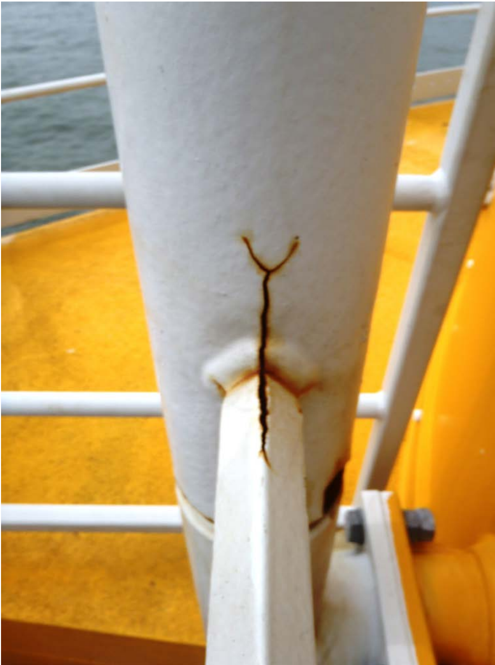
Figure 9. Cracks in a coating film caused by inner tensions in the coating film from excessive DFT.
