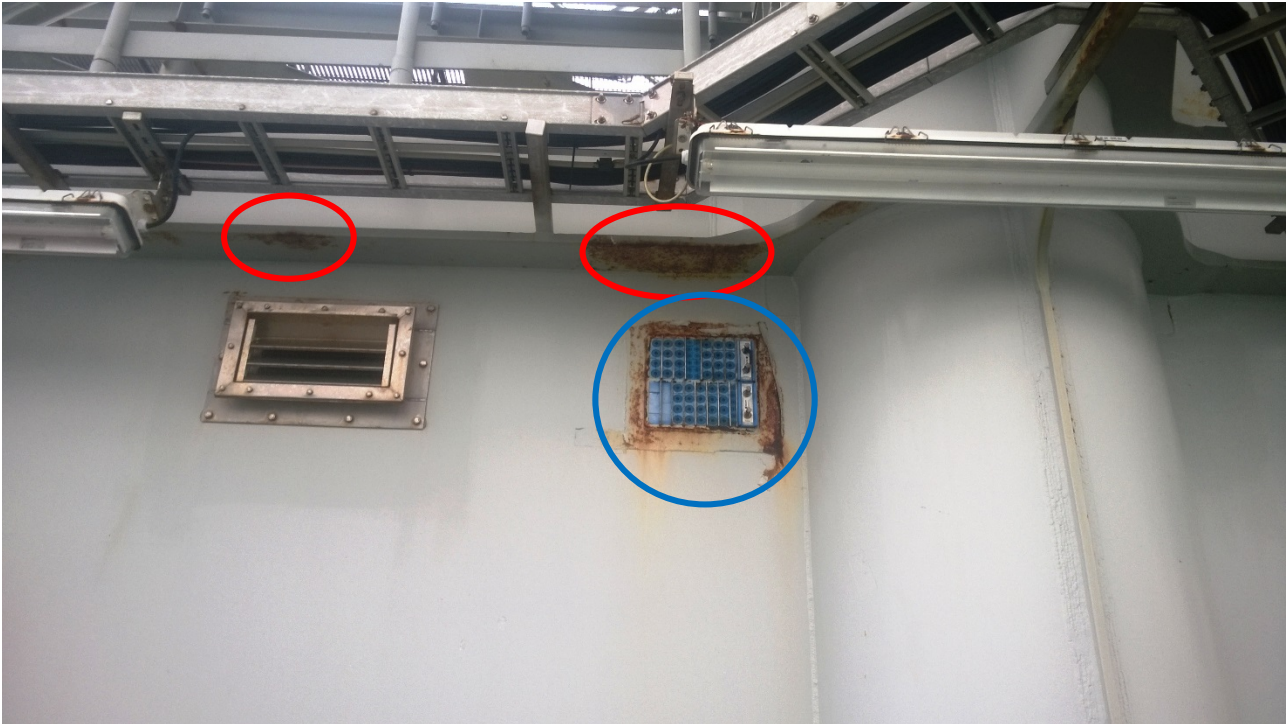
Figure 7. Offshore transformer station. Two typical faults in the surface treatment process that initiate corrosion attacks: Red circles: Lack of rounding of edges (chamfering) on part of the steel bar. Blue circle: Poorly mounted and painted light accessory after installment of the station. See also the intact ventilation duct on the left hand side, which has been mounted correctly during the manufacture of the station.
