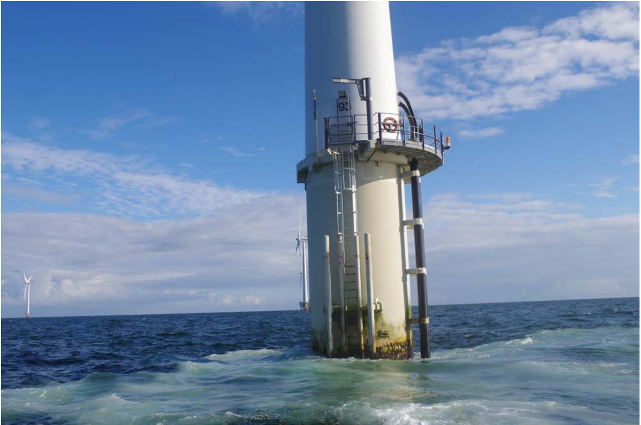
Figure 5. HR 1 in 2015. TP painted with the high DFT solvent free epoxy system 1000-1100 \mu\text{m} after 14 years of service. The protection of the coating system is intact.
