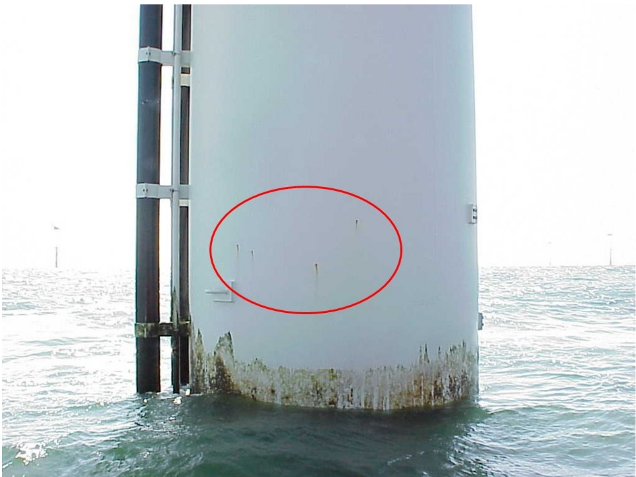
Figure 2. Horns Rev 1. Pinpoint corrosion on TPs with the lean two-coat epoxy system after two years of service.
