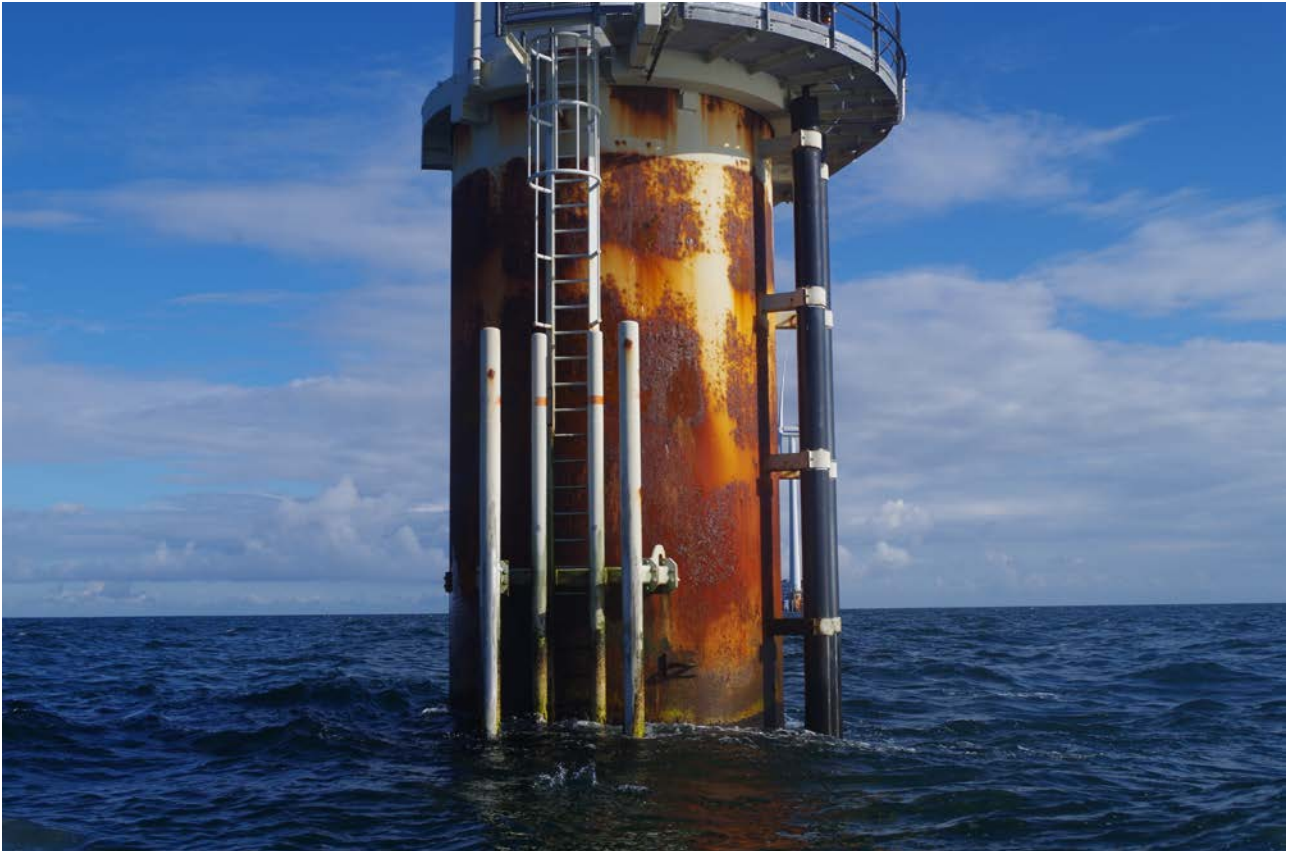
Figure 6. HR 1 in 2015. TP painted with lean and permeable coating system after 14 years of service. Compare the corrosion progress with Figure 2.
