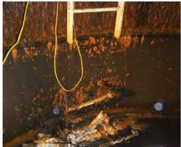
Figure 1: Corrosion inside offshore wind turbine foundation
