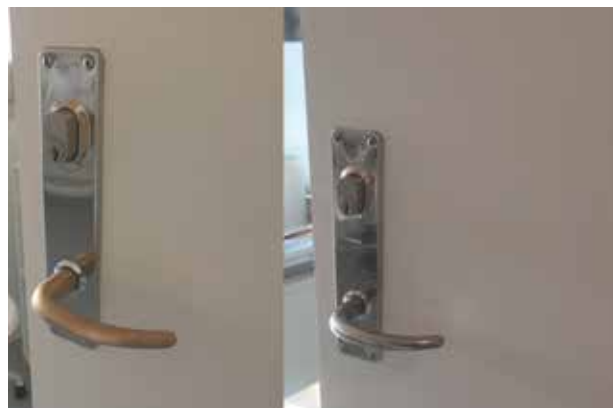
Coated and uncoated door handles during the field test in Kvistgaard, Denmark.
