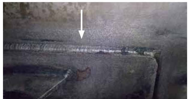
Figure 2: Image from the current vessel with a rough appearance in the vicinity of a weld. This could be an early indication of pitting corrosion.
