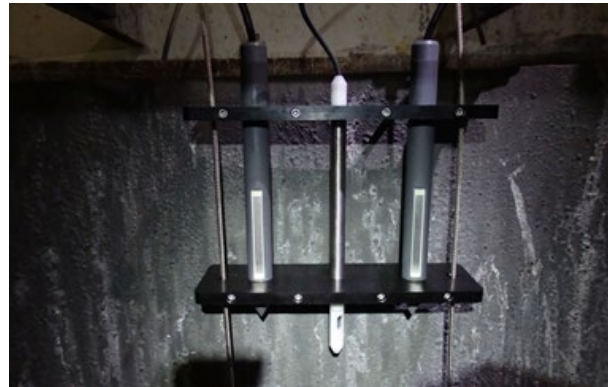
Figure 7: An ER probe installed on the monopile wall.
