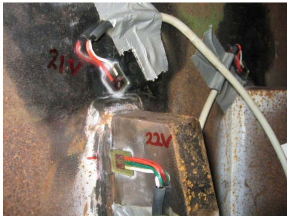
Figure 9. Strain gauge sensors close to bracket. MPI has also been conducted to check for cracks at welds.
