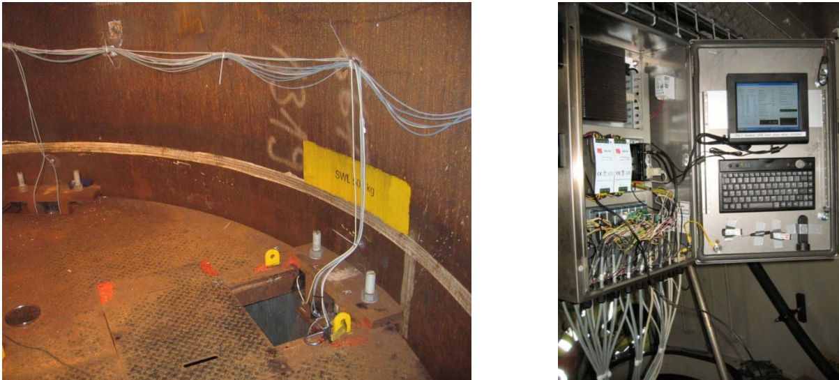
Figure 7. Installation of cables and equipment for monitoring of large number of sensors. Cables continue below the platform. The cabinet with a complete data acquisition system mounted just above the airtight deck.
