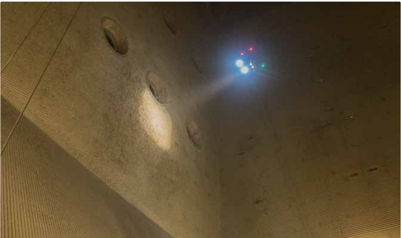
Drone inspection of boiler. Equipped with lights, the drone is well suited for inspection of spaces with little or no light.
