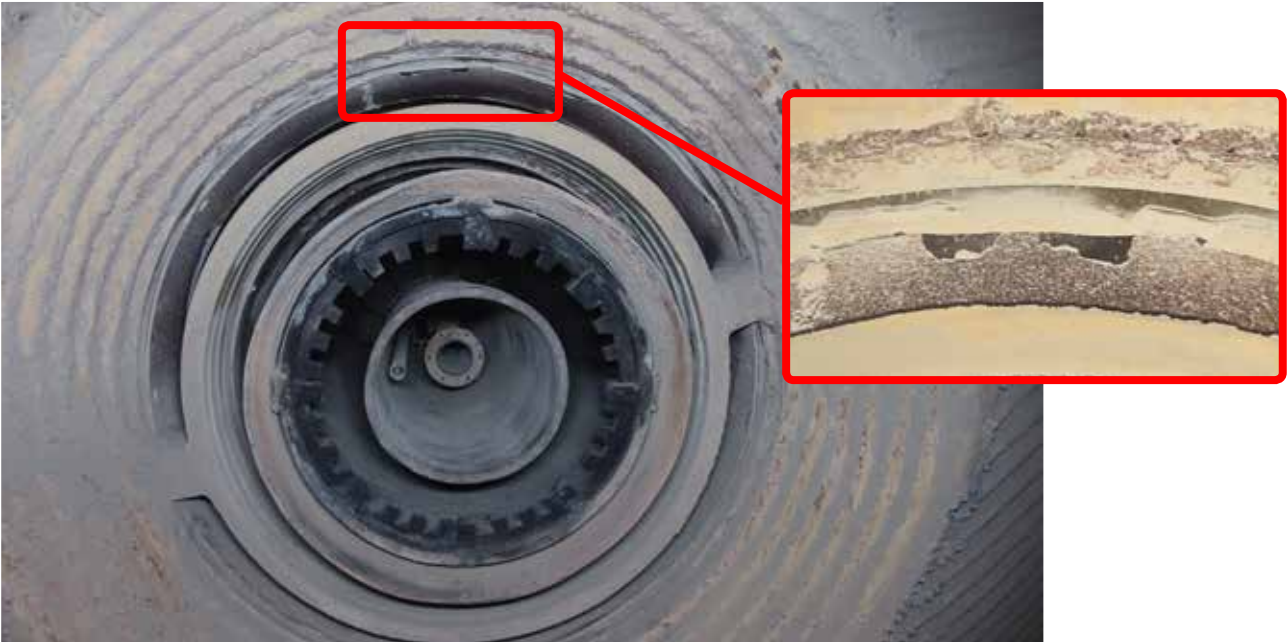
Cracks in boiler detected by drone inspection.
